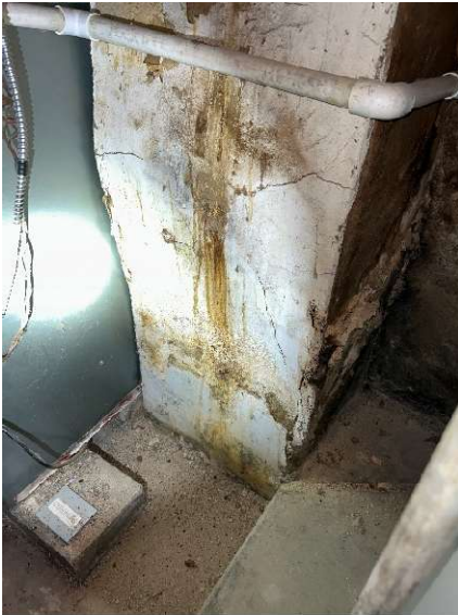
Damaged chimney base
