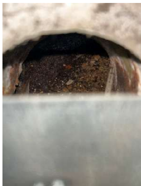
Corroded debris in the cleanout
