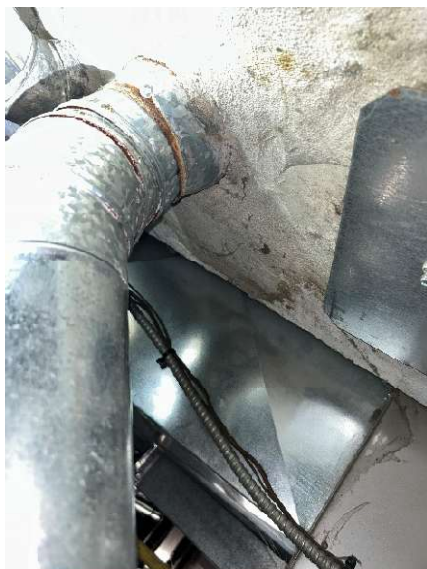
Corroded chimney seams
